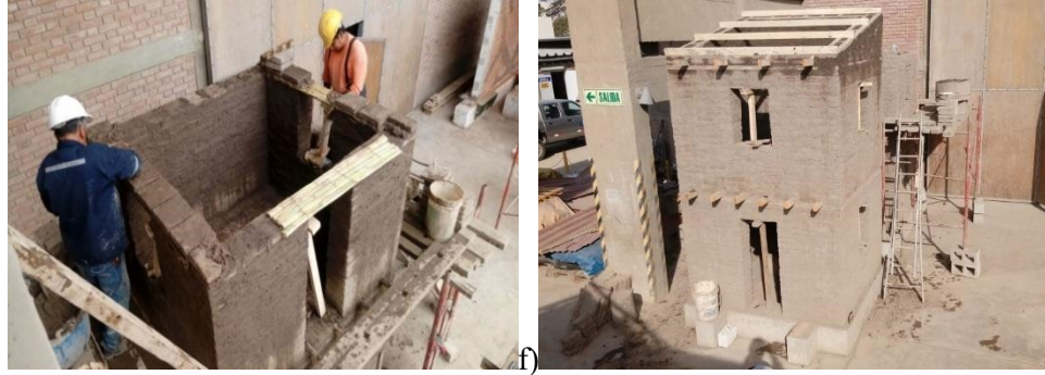
291 e) f) 292 Figure 9 (Continuation). Construction process sequence of an unreinforced model. a) b) construction of 293 first level walls; c) and d) installation of the wood crown beam and wood beams; e) lintels of doors and 294 windows (made of cane rods tied with wire), f) finished model (before roof tiles placement). 295
