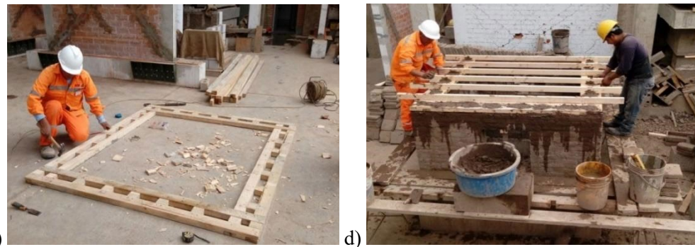
287 Figure 9. Construction process sequence of an unreinforced model. a) b) construction of first level walls; 288 c) and d) installation of the wood crown beam and wood beams; e) lintels of doors and windows (made of 289 cane rods tied with wire), f) finished model (before roof tiles placement).
