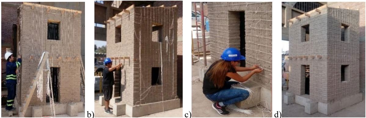
318 a) b) c) d) 319 Figure 11. Sequence for the reinforcement process: a) installation of vertical ropes; b) installation of 320 horizontal ropes; c) joining of inner and outer meshes; d) reinforced adobe model. 321
