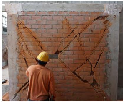
(a) Cracks opening
