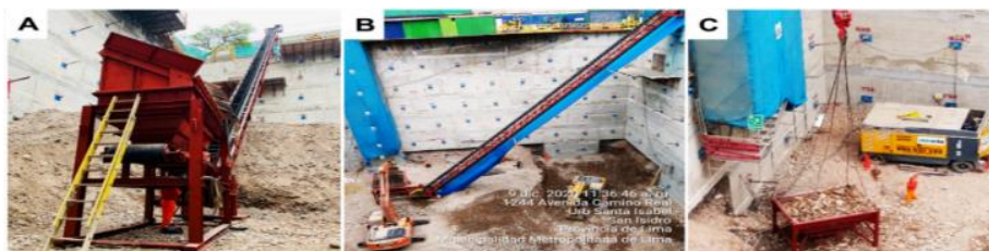
Figure 6. Operation of the conveyor belt and bucket crane.
