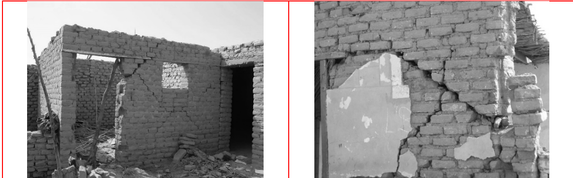
Fig. 2 Typical in-plane damage in adobe walls.
