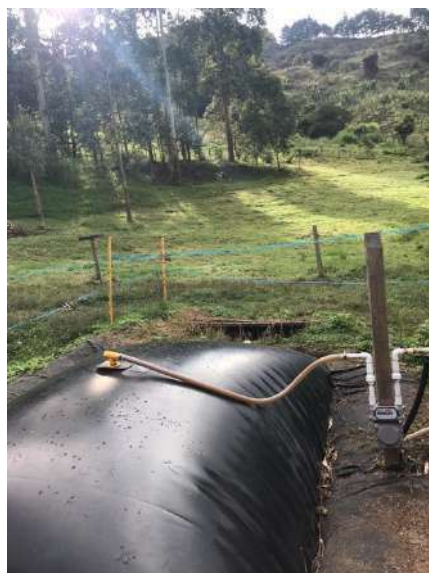
Figure 1: Psychrophilic tubular low-cost digester implemented in Colombia. Source: Personal archive.
