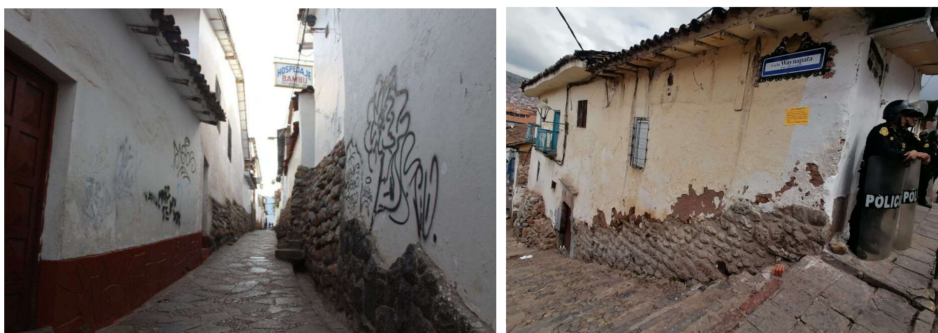
Figure 1. Viceroyalty architecture of Cusco with lime plaster coatings. Note: Examples of facade deterioration on heritage buildings in Cusco’s historic center. Graffiti, plaster detachment, and patches made with incompatible materials are visible issues linked to the limited access to lime for traditional maintenance because it is a regulated input in Peru.
