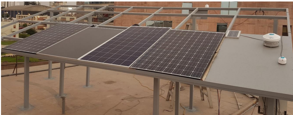
Figure 1. Photovoltaic Research Laboratory for the monitoring and characterization of PV modules and environmental sensors, localized on the roof-top of the Physics Section at the PUCP.
