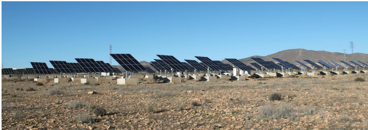
Figure 1. View of the 109.4 kW photovoltaic generator.
